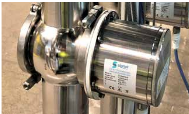
Transfer pipes with TurbiGuards installed inline
