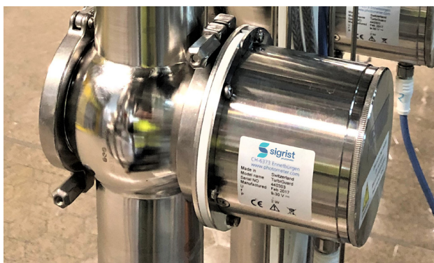
Transfer pipes with TurbiGuards installed inline
